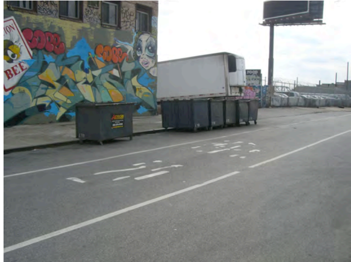
Figure 3. Deteriorated speed limit pavement marking, Boone Avenue, Claremont
