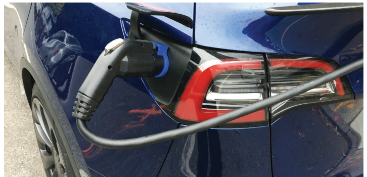
24-hour EV charging at the recently installed FLO charging station at 99 Prospect Park West, between 5th and 6th Streets
